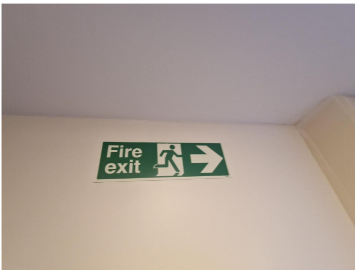
Escape route signage displayed.
