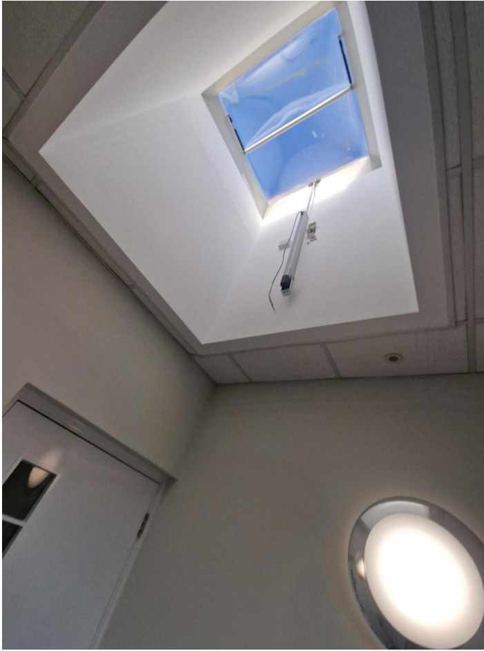
Smoke ventilation installed.
